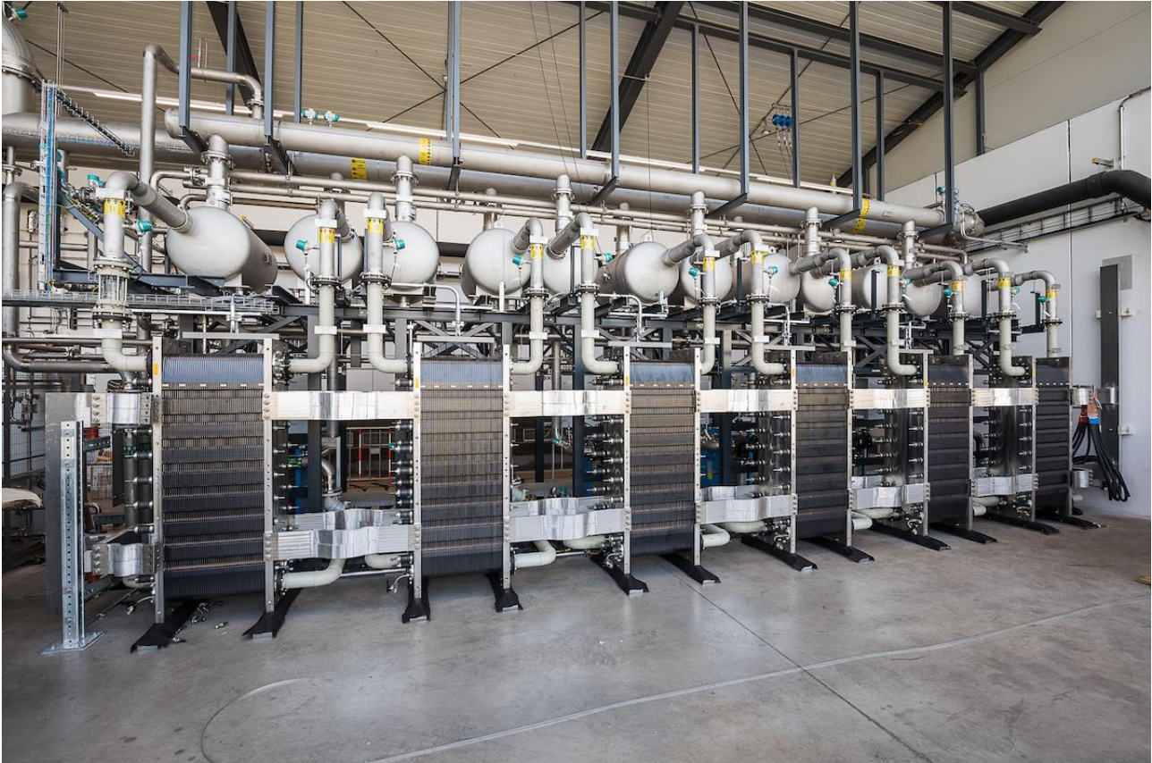
H2FUTURE PEM Silyzer 300 electrolyser (source: © voestalpine)
